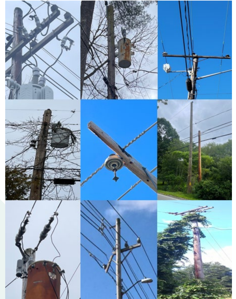
Defects in the distribution system
