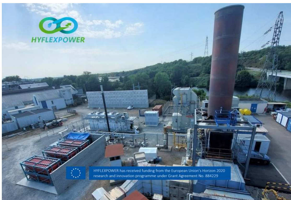
HYFLEXPOWER, the first fully integrated power-to-H 2 -to-power demonstrator with an 100% hydrogen gas turbine
