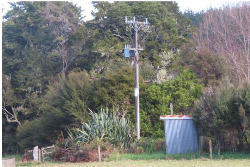
Figure 4 - Pole-top distribution substation
