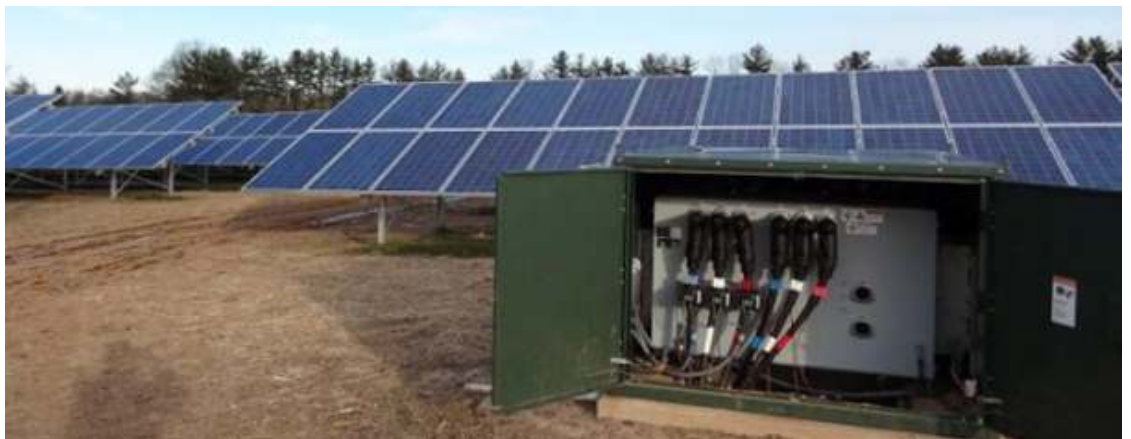
Medium Voltage padmount switch
