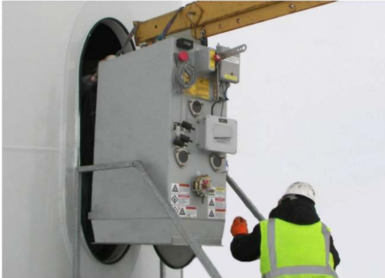
Offshore wind tower switch
