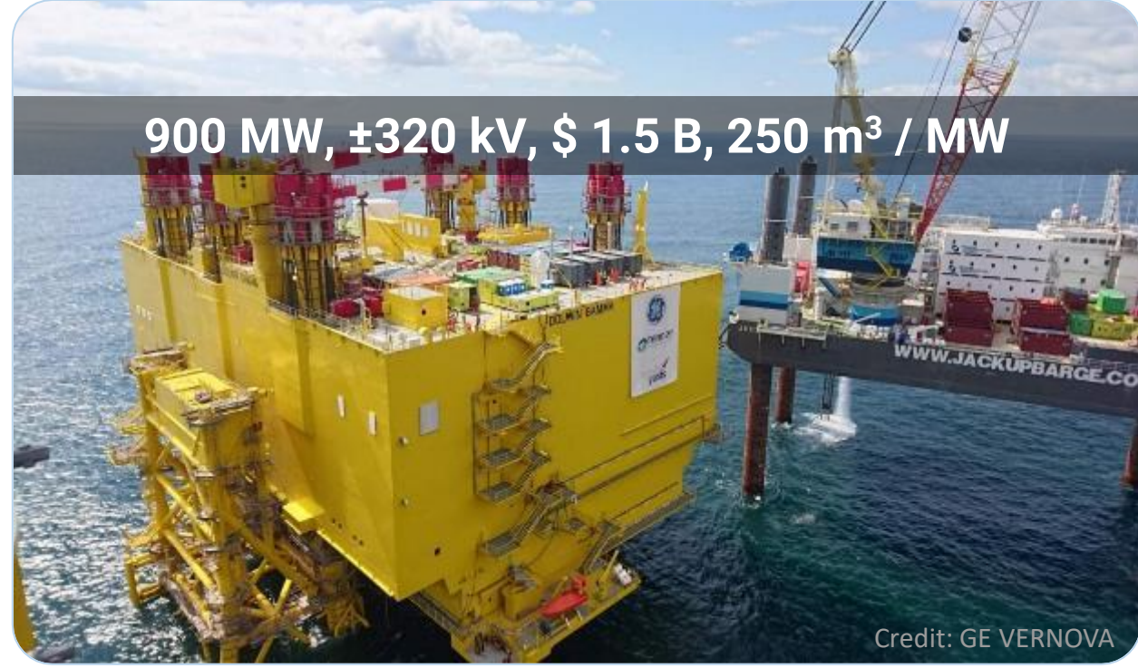
Dolwin-3 Off-shore HVDC Station (2017)
