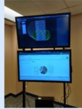
Network Control/Security Operation Center
