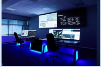
Energy Control Center
