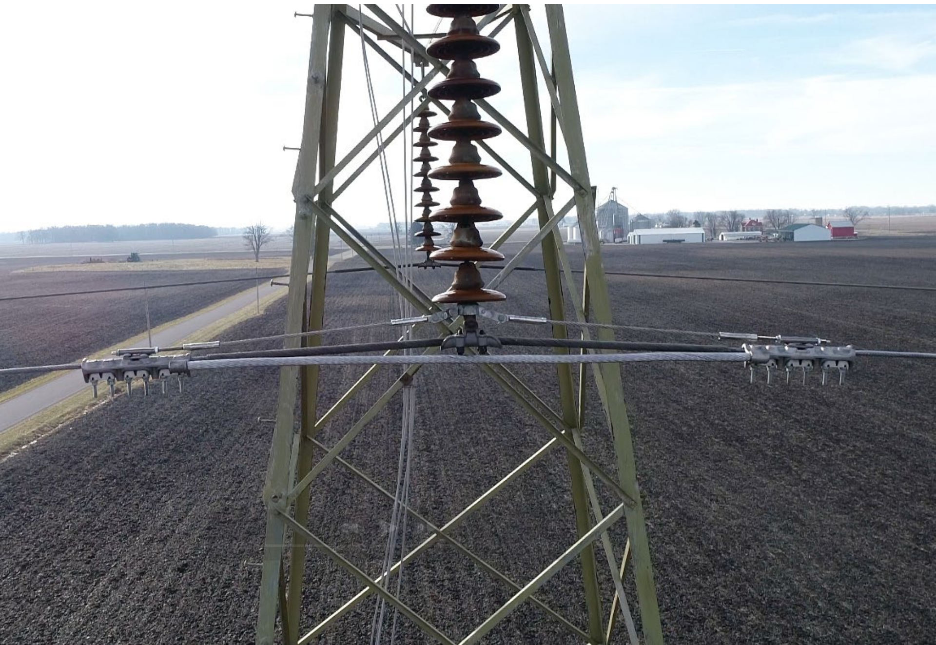
Typical Ball Cap application, 477 Hawk with armor rods – broken strands under rods.
