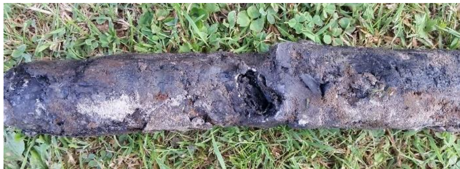
Figure 4: Weak spot in the PILC cable caused by small stone.
