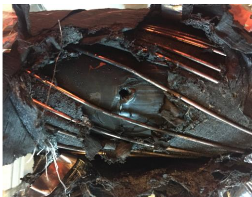
Figure 4: Dielectric failure of XLPE cable with electrical puncture through outer semicon screen. Much or all of the root cause evidence is destroyed by the withstand test fault.
