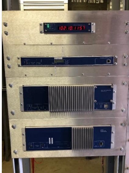
Figure 5: FCP substation IEDs
