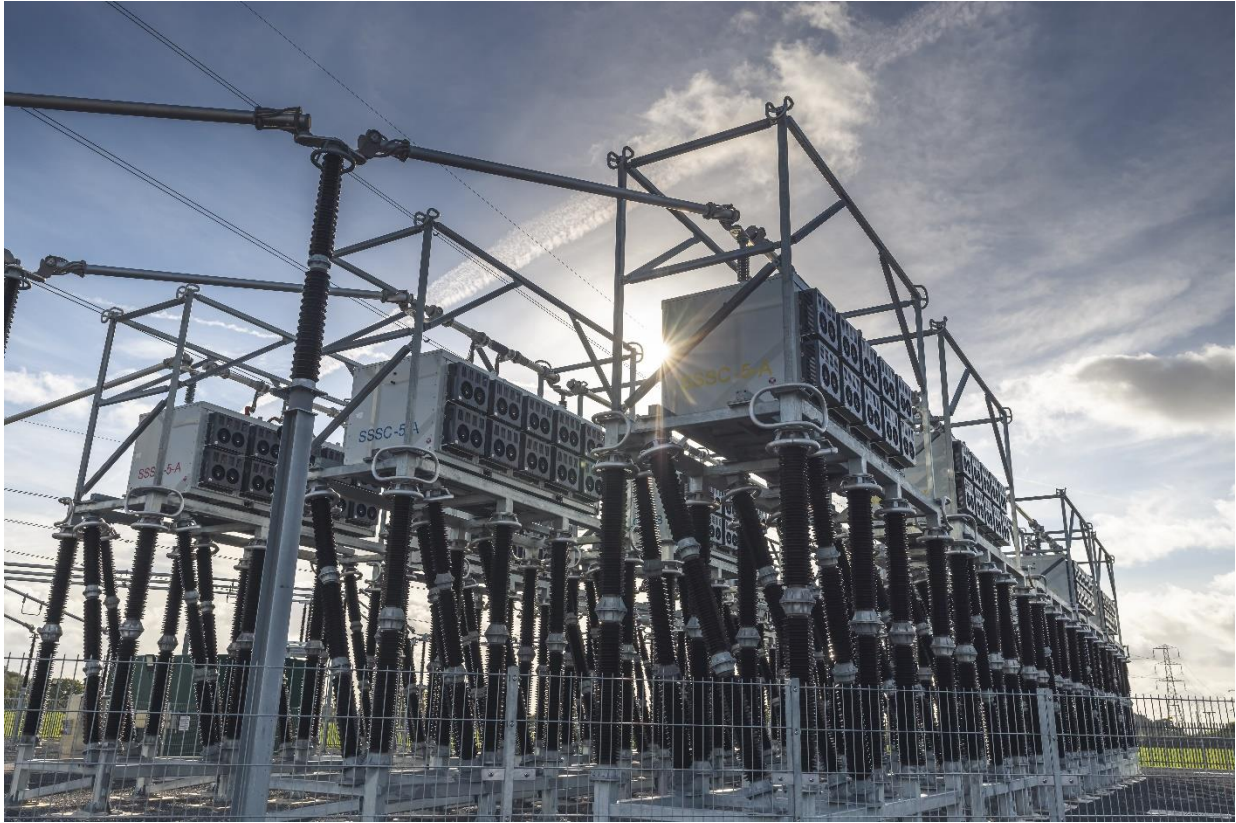
Figure 7: M-SSSC installation on National Grid's system in the United Kingdom
