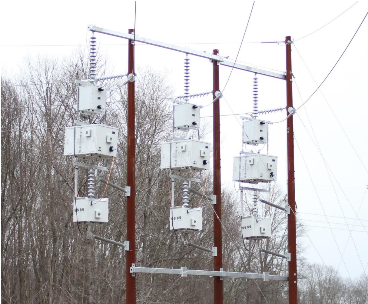
Figure 6: M-SSSC Phase Two Pilot Installation on Central Hudson's System
