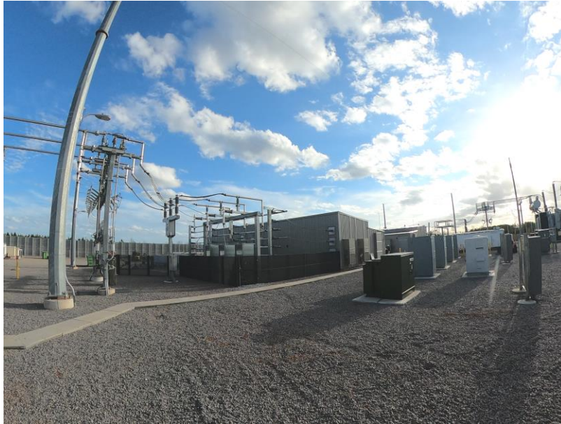
Fig. 7. Rawlings #1 STATCOM control building, medium voltage bus, reactor yard, and station service equipment(foreground); Rawlings 2 STATCOM medium voltage bus and control building (background).
