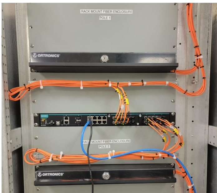
Figure 4: An image of the Moxa switch enclosure and fiber connections (orange) located in the control room. The blue ethernet cord connects directly from the Moxa switch to an engineering laptop for data exchange.
