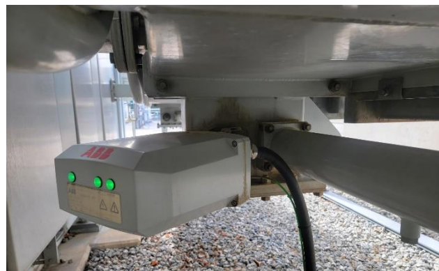
Figure 2: Close-up image of the DGA CoreSense Sensor Head installed on the cooler drain valve of the transformer.
