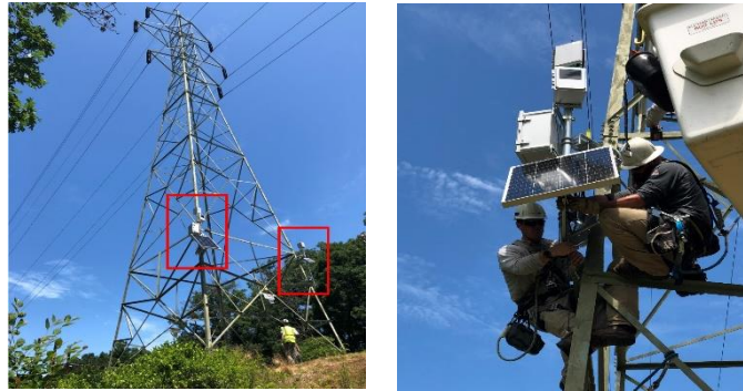
Fig.1 Photograph of the structure and installed equipment (Tech A)
