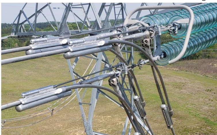
Photograph above on a tri-bundle 500kV installation
