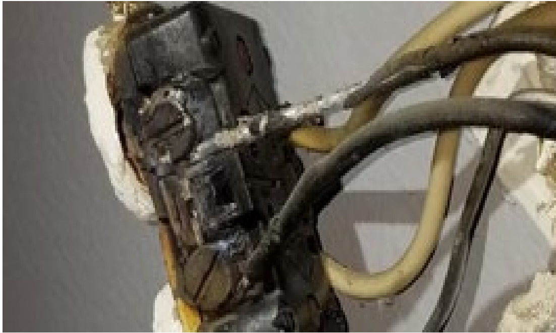
Damaged Wall Outlet
