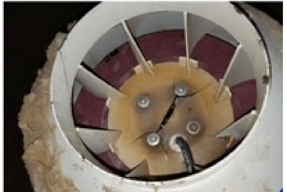
Failing Radon Pump
