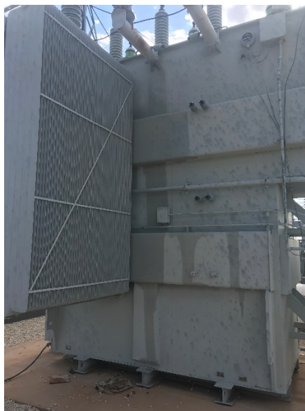
Figure 6: 138kV to 69kV Autotransformer Oil Leak [5]
