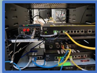
LTE gateway access endpoint equipment
