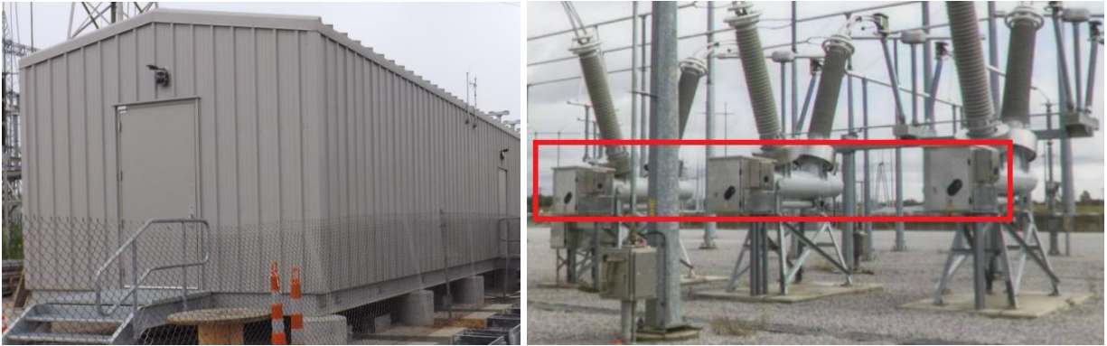
Figure 2: DICM and circuit breaker control cabinets (examples)
