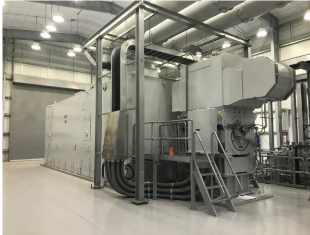
Figure 5: Synchronous condenser installation with a pony motor
