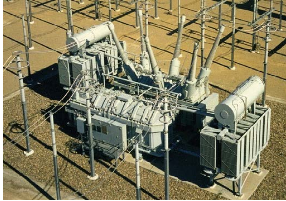
Phase-shifting transformer (PST)
