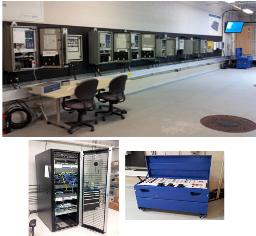
Figure 6 Recloser controls set up (up), data concentrator and networking equipment (lower left) and fault tester (lower right)
