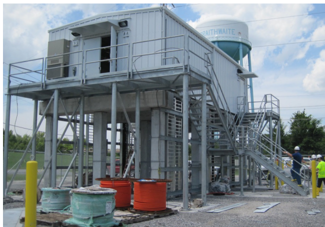
Figure 1 – Elevated control house resists flooding
