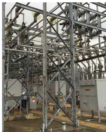
Figure 2 – Joliet Sub, site of storm flooding, now process bus test site.
