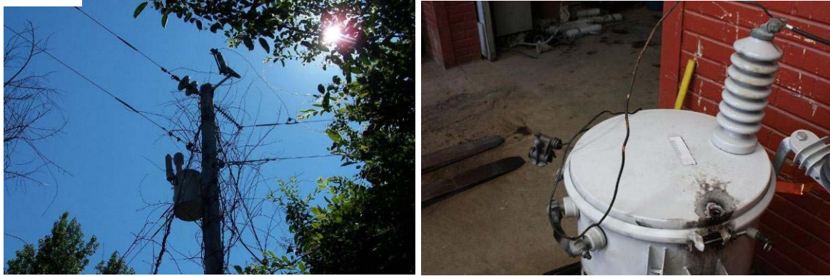
Figure 2: Pole-top transformer a) with vines atop pole, b) after removal from service, with hole visible.
