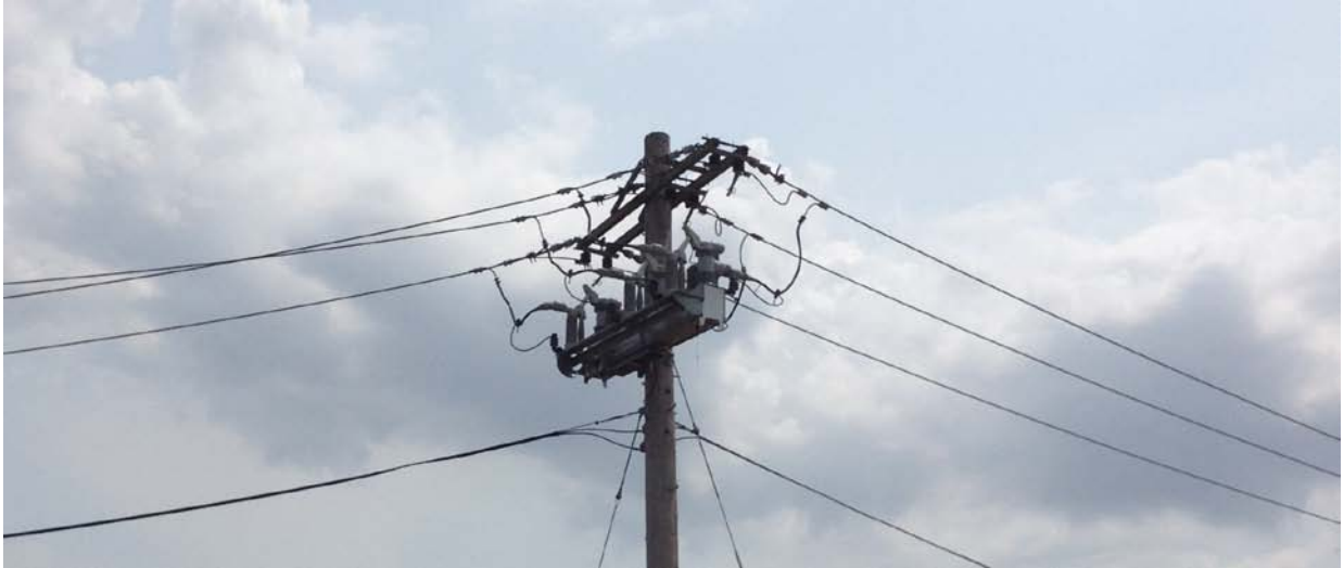
Figure 1. Example pulsecloser installation on Ameren’s system
