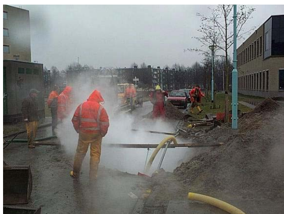
Photo 1 'freezing of 36/50kV fluid filled cable in urban area'
