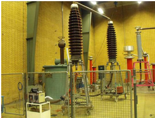
Photo 4 '87/150kV LPOF cable injected with PFT type test loop'
