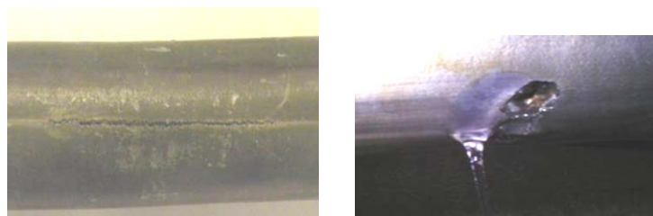
Photo 6 'typical defects of lead sheathed LPOF cables after ageing'
