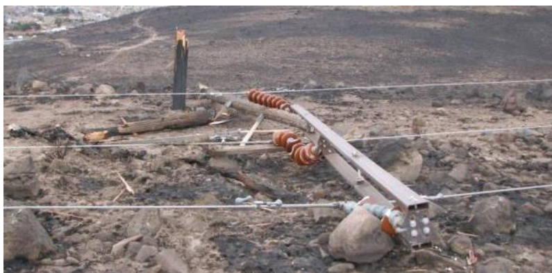
Figure 7 – ACCC conductor undamaged after support structures burned to the ground
