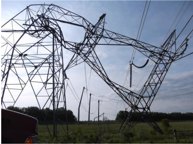
Figure 10 – downed lattice structure that dropped its double circuits lines onto an underbuilt ACCC circuit without damaging the ACCC wires
