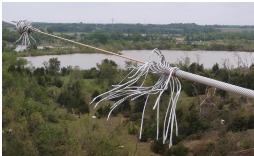
Figure 9 – ACCC conductor damaged by EF5 tornado
