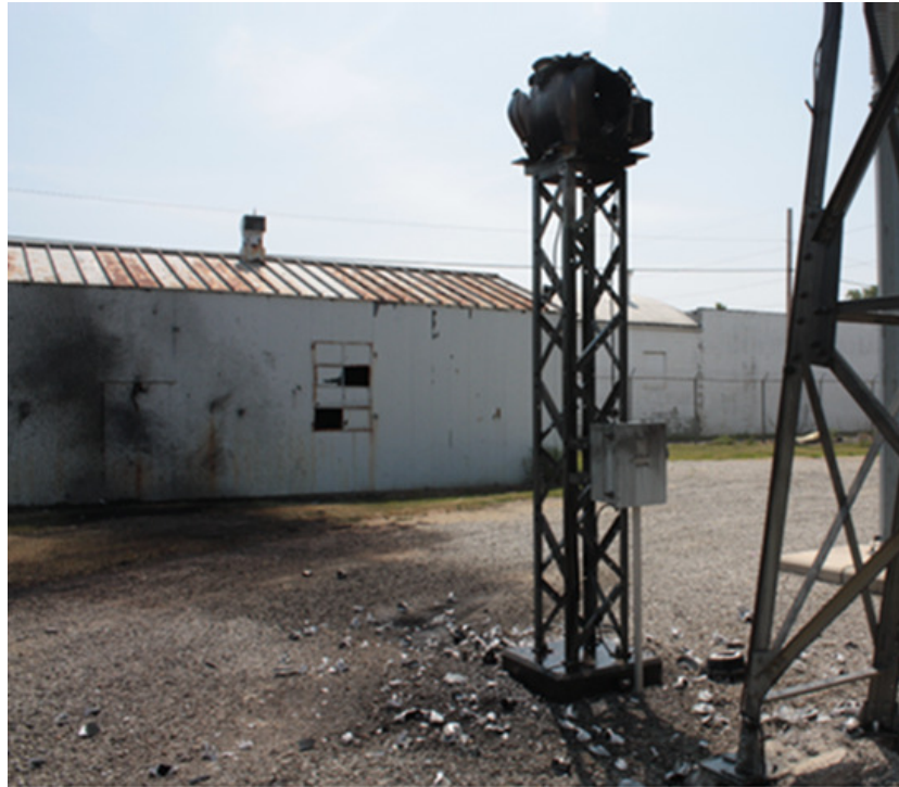
Figure 1. CCVT Violent Failure Caused Explosion Damage in one of AEP Substations
