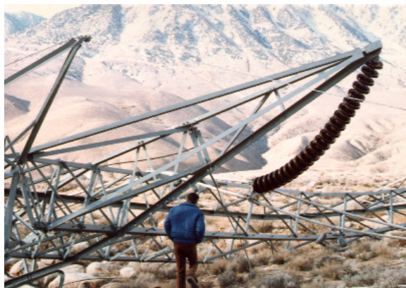
Figure 1: One of 16 cascaded 500kV DC Towers collapsed at the Los Angeles Department of Water and Power (LADWP) in 1988 due to High Winds
