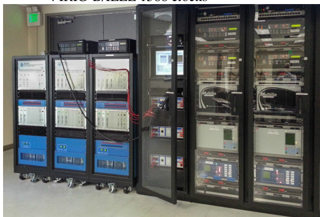
Figure 2 View of the PoC facility
