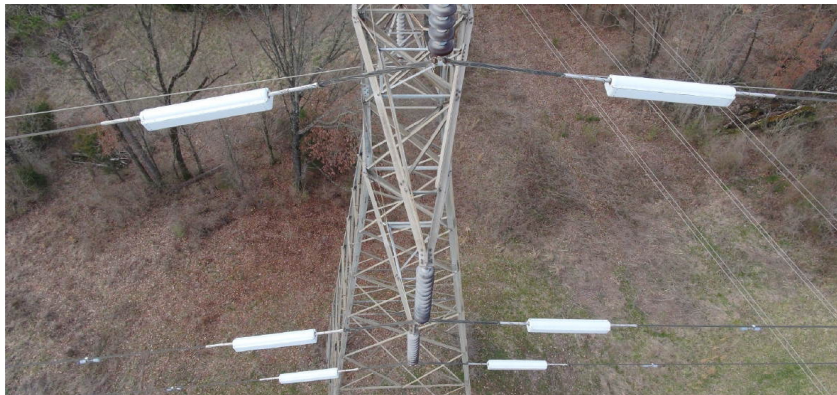
Figure 4- Power Flow Control Devices Installed on High Voltage Line
