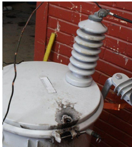
Figure 2: Transformer damaged by repetitive fault.
