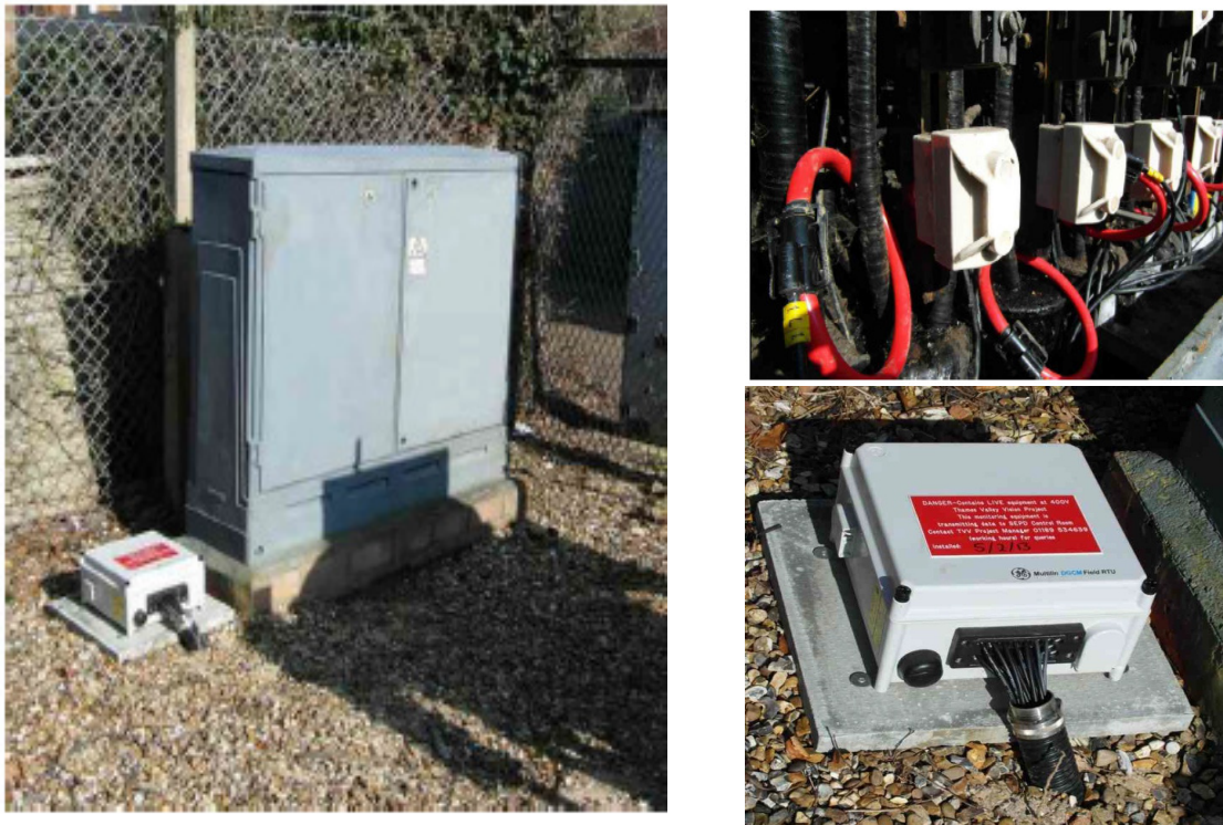
Figure 5 LV Monitoring node installation at distribution substation [Courtesy: SSEPD]
