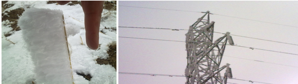
Figure 1. Accumulation of snow and ice on the lattice tower, insulators and conductors
